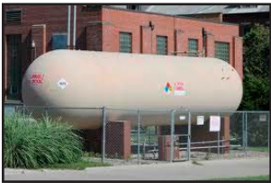
Figure 22-35 LPG (Propane) Tanks
