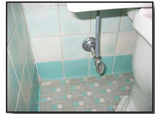
Figure 22-44 Localized Water Valve
