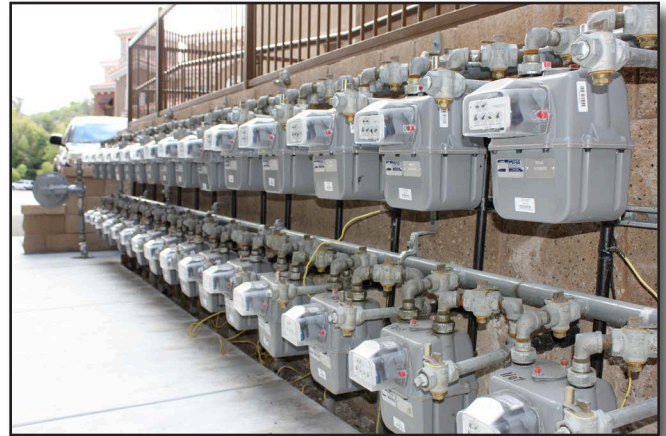
Figure 22-42 Multiple Gas Meters Serving a Large Apartment Complex
