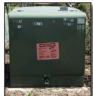
Figure 22-8 Live Front Terminator Box (above 2 images)
