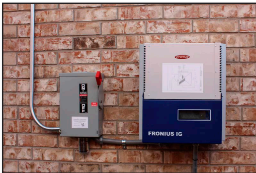
Figure 22-29 D.C. Power Disconnect and D.C. to A.C. Inverter
