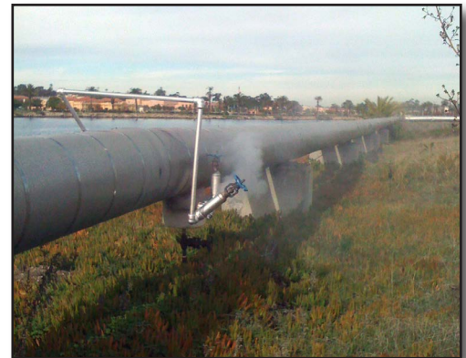
Figure 22-56 High Pressure Steam Pipe
