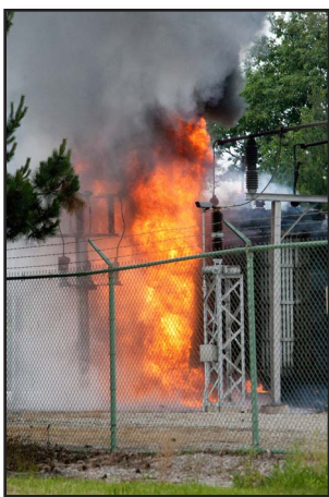
Figure 22-14 Electrical Fire in a Substation
