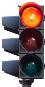
Figure 22-15 Traffic & Street Lights are Considered High Voltage
