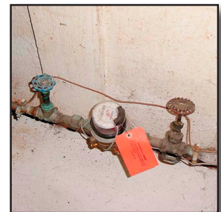
Figure 22-45 Water Meter with Globe Valves
