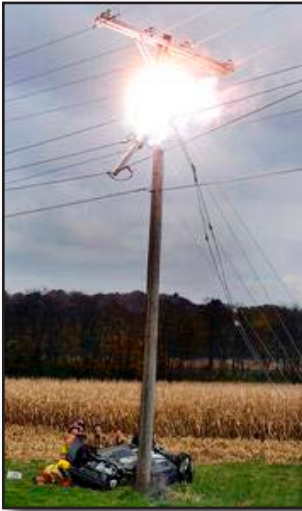
Figure 22-17 Pole Fire - Stay back 2 pole spans
