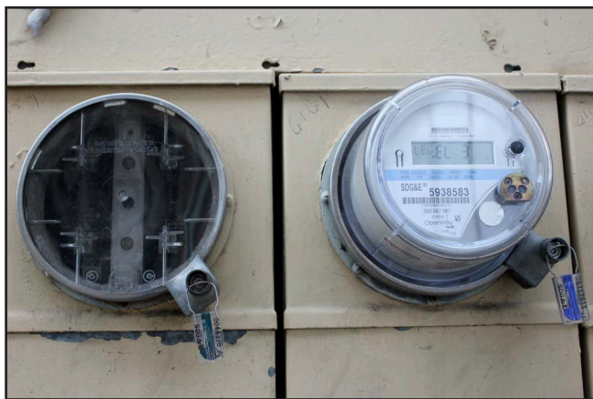
Figure 22-26 The service panel on the left has had it’s meter removed and locked by SDGE.
