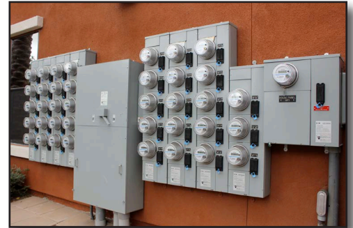
Figure 22-22 Multiple Metered Panels
