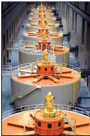
Figure 22-1 Hydroelectric Dam & Generators
