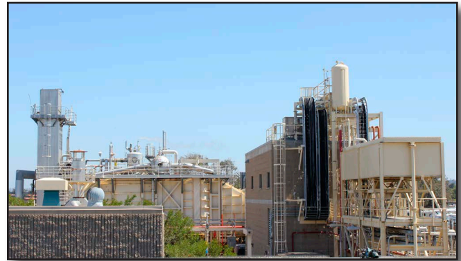
Figure 22-55 Steam Power Plant at NTC San Diego
