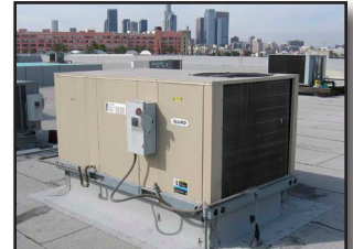
Figure 22-57 Commercial Roof Mounted HVAC
