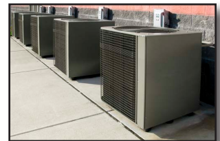
Figure 22-58 Residential AC Units
